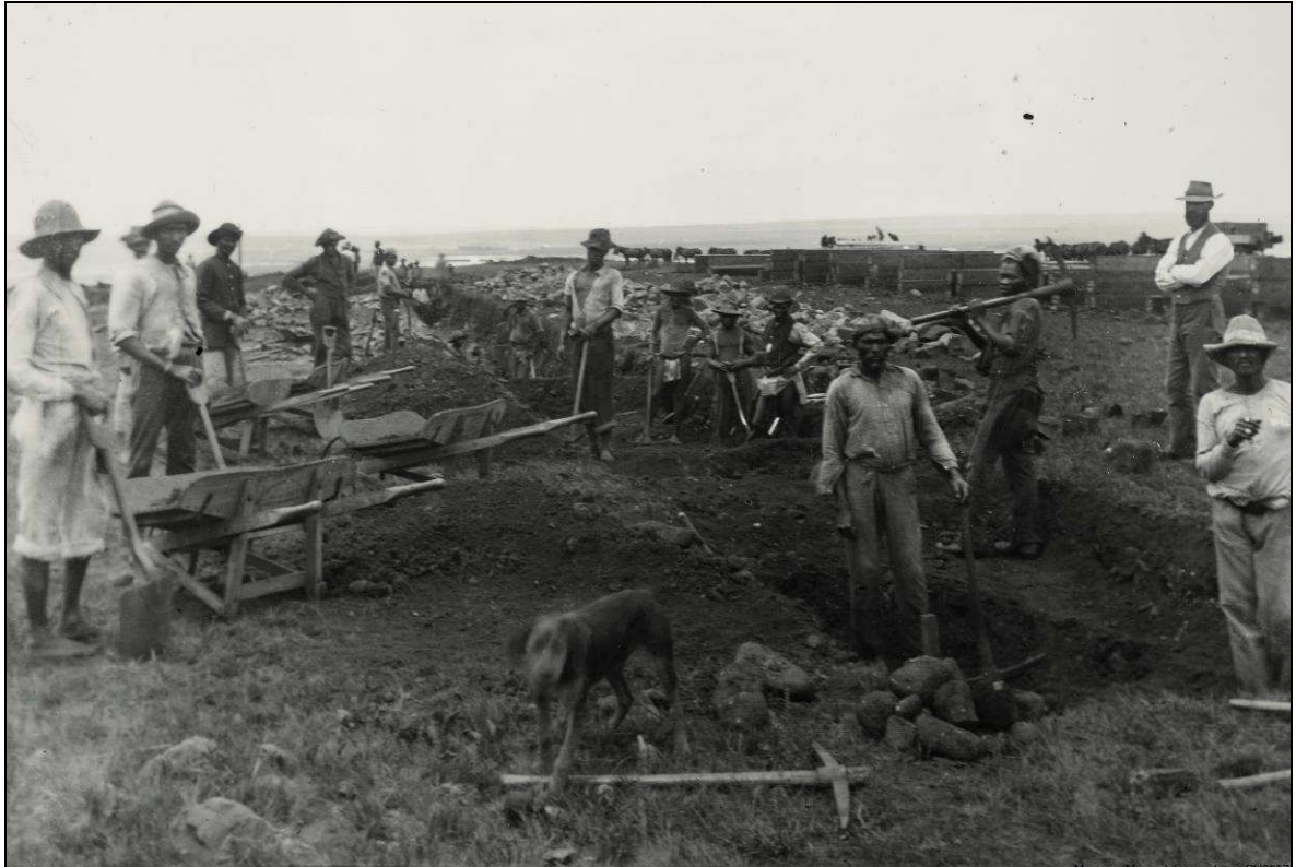
Figure 2 Undated photograph of early mining activities at Driefontein Consolidated Mines Limited (Museum Africa, Photographs, PH2007-33259). During the early years all gold mining activities were undertaken on the surface.
