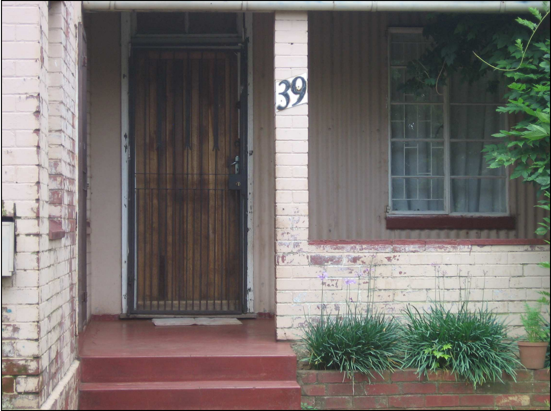
Plate 12 The front veranda of one of the existing units from the old married quarters. This unit is number 39. The corrugated iron sheeting on the walling next to the door can clearly be seen. As discussed elsewhere the corrugated sheeting must have formed part of the original structure.
