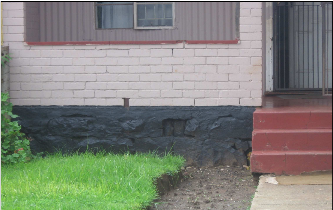
Plate 13 A section of the front elevation of another existing unit from the old married quarters. The original structure's corrugated iron sheeting and stone foundation can clearly be seen.
