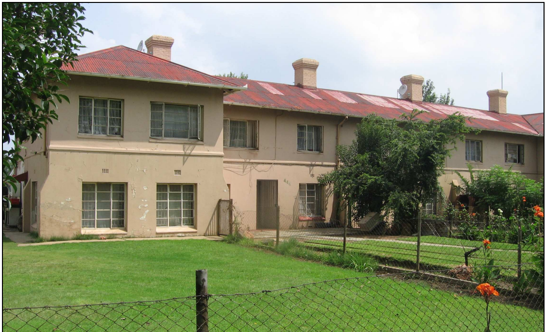
Plate 15 General view of the northern elevation of one of the units indicating the new steel frame windows that replaced the casement windows of Baker.
