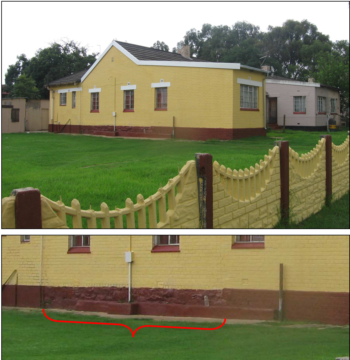
Plate 9 Side elevation of one of the existing buildings from the old married quarters. The enlarged image (bottom) clearly shows the original stone foundation. The stone foundation is marked in red.
