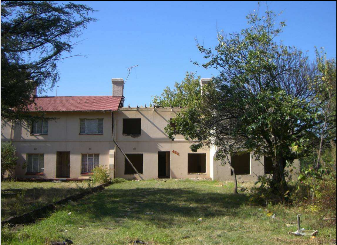
Plate 38 This image taken before or during 2007 appears to show the new married quarters building known in this report as Building 6.
