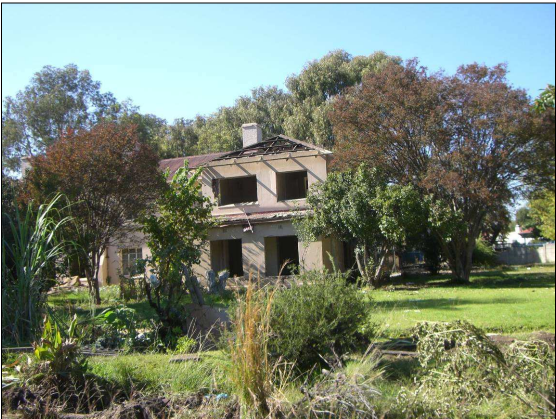
Plate 43 Another image of what appears to be Building 7. This photograph was must have been taken after the previous one.
