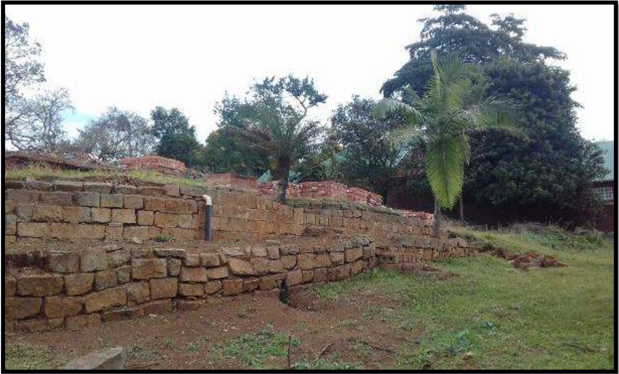
Plate 1. The retaining walling below the foundations of the demolished house. These large blocks created terracing leading to the demolished house. These large, undressed blocks are quite typical of the older properties in the KZN Midlands. One can see just above the stone walling bricks which were obtained from the house stacked up around it. Old cycads can be seen to the right of the photo. Photo: Frans Prins.
