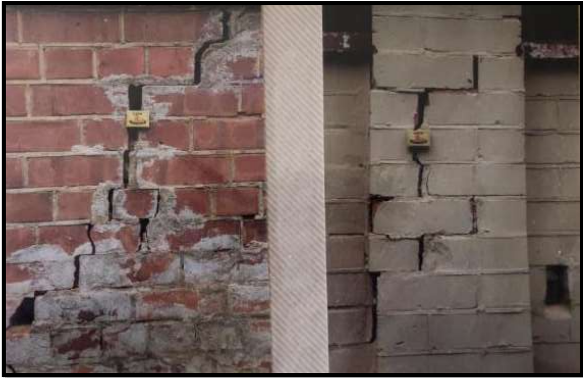
Photo 12. These are photos of a brick wall in which there are large cracks. These photos were provided by Mr Mohammed Moosa, stating that they are of the walls of the house at 12 Craigie Drive. Photo: courtesy Mr Mohammed Moosa.
