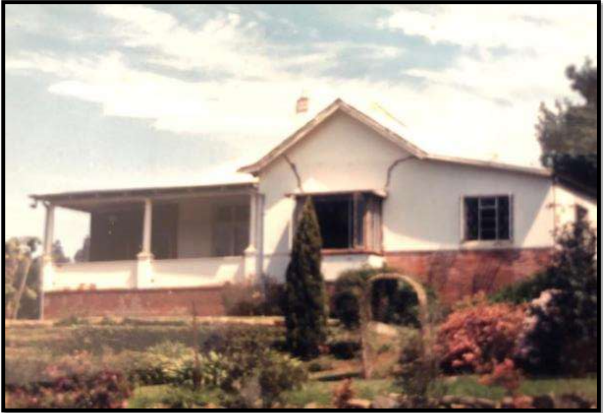
Plate 11. In this photo the Victorian-Edwardian pitched roof, high chimney, deep columnaded verandah and red brickwork are all apparent. While perhaps not an aesthetically pleasing house, this house is very typical of farmhouses in this region. The cracks in the walls of the house are also very apparent. Photo: courtesy Mohammed Moosa.
