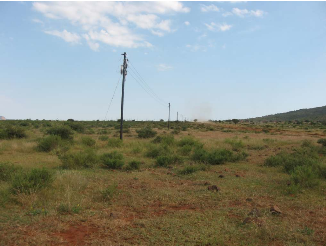
Photo 2: View of the power line from the south.
