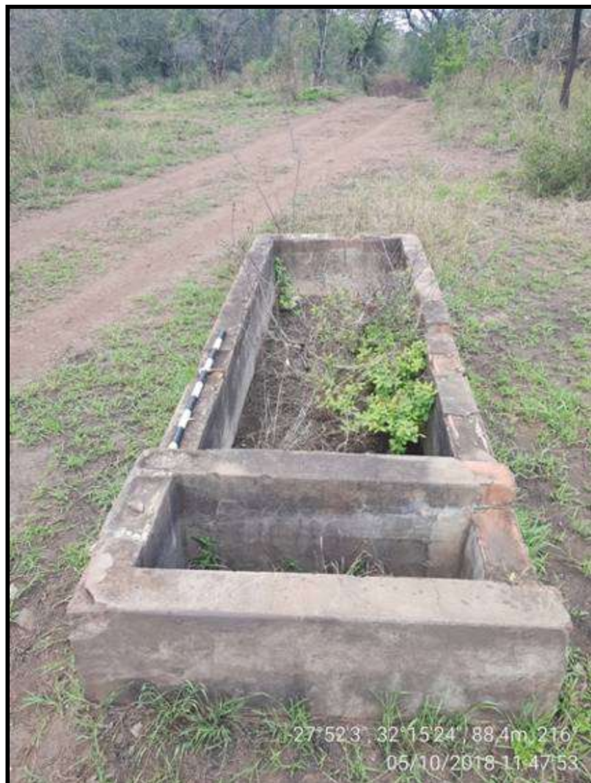
FIG. 145: WATER TROUGH AT WP661
