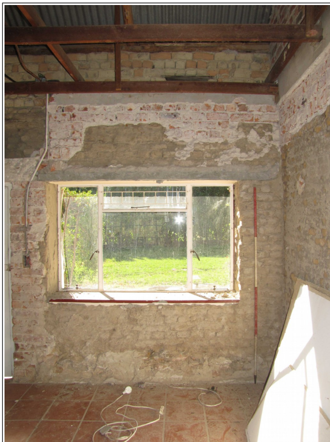
Plate 4: Western elevation. Phase 5 window 05 inserted into sun-dried brick of wall 02. View to the north-west, 2.0m scale.
