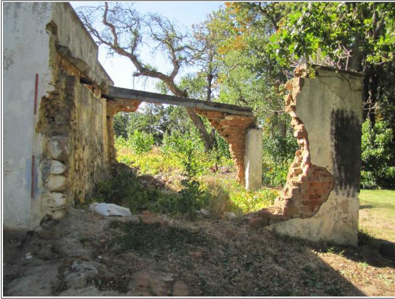
Plate 4: 'Dilapidated Structure' at the north end of West Barn.
