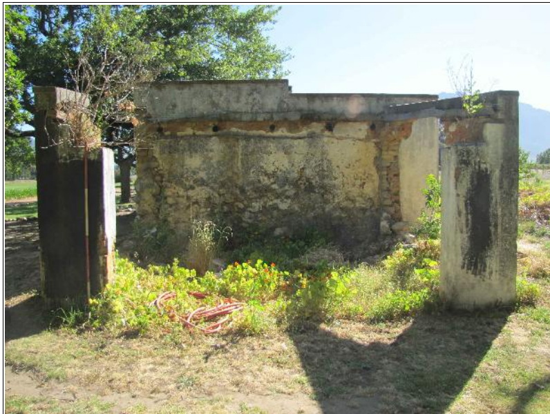
Plate 5: Photograph showing double-doorway to north elevation of 'Dilapidated Structure'
