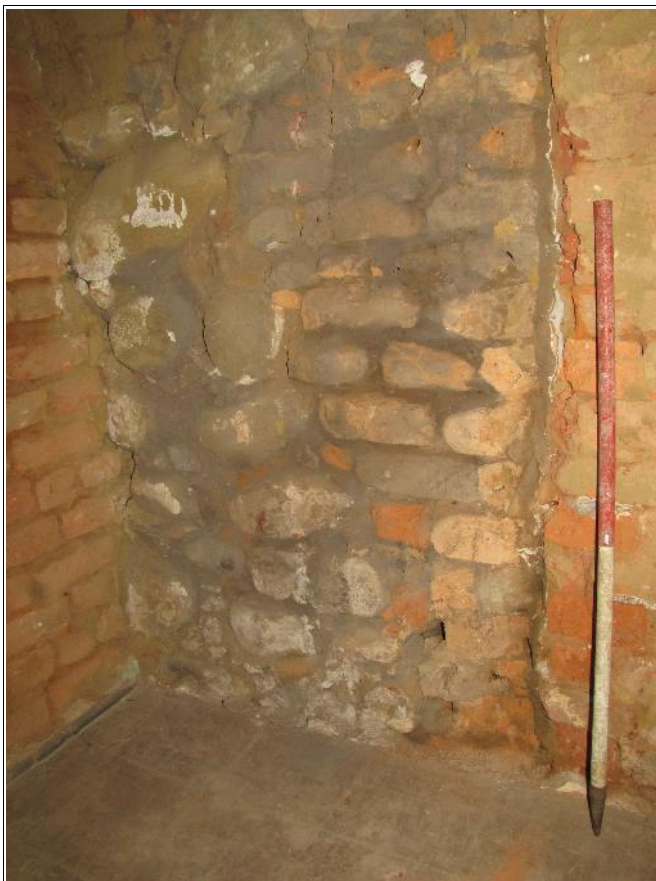
Plate 3: Section 2 showing plaster on jamb of doorway 18.
