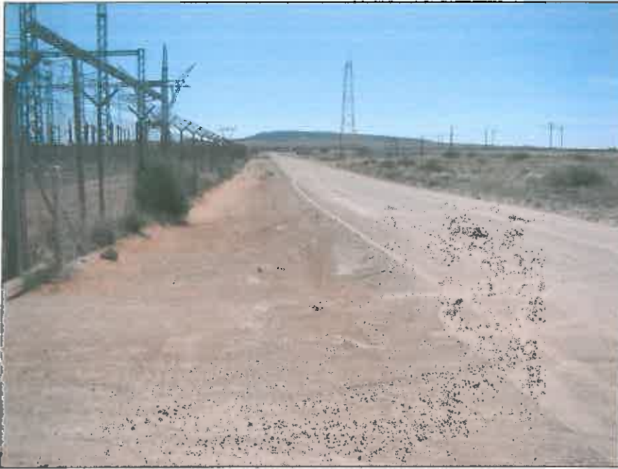
Fig.2 Garona substation on the Sishen-Saldanha railway line.
