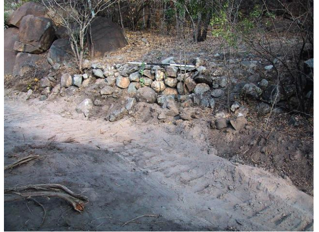
Fig 8. Road damage to stone wall, site 1
