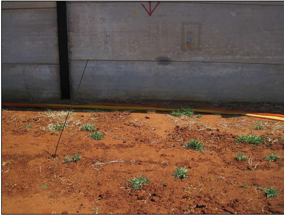
Figure 14: IVN_PGS_22_04 with the barricade partially removed on arrival before excavation work began
