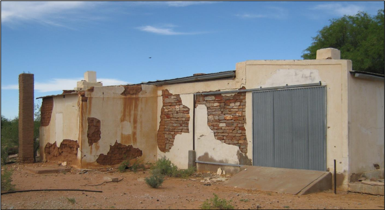
Figure 29: Dilapidated structure at the farmstead ay waypoint 526.
