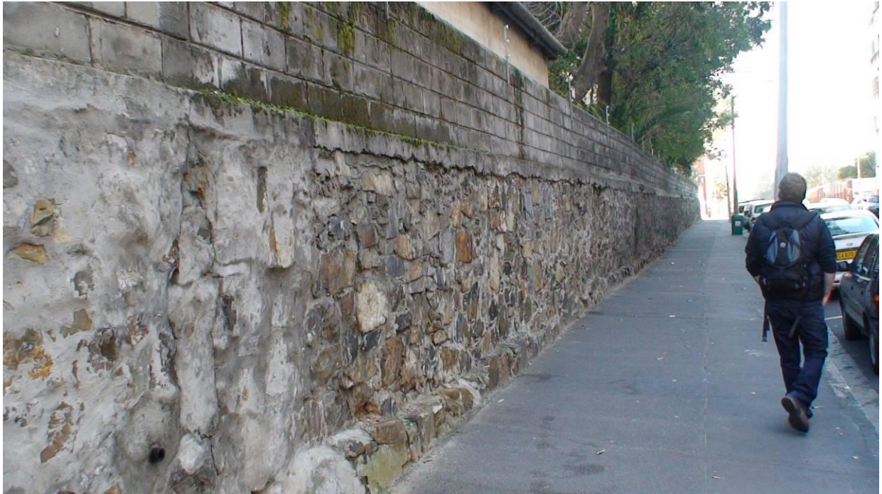
Figure 16. The old cemetery wall of the Military/Scottish cemetery is one of the oldest structures in Cape Town. Soil levels within the grounds reach the top of the bluestone wall, hence the cement block height extension.
