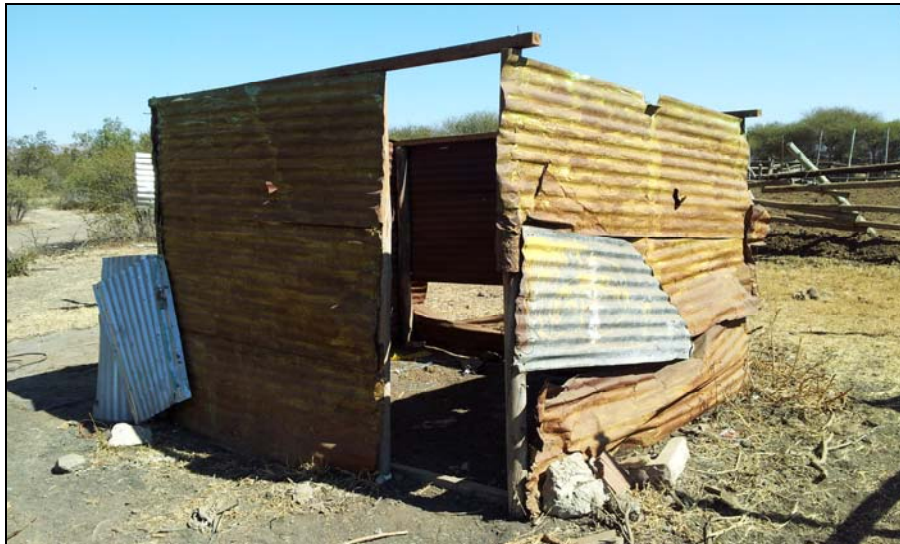
Figure 10: The remains of a dilapidated shelter
