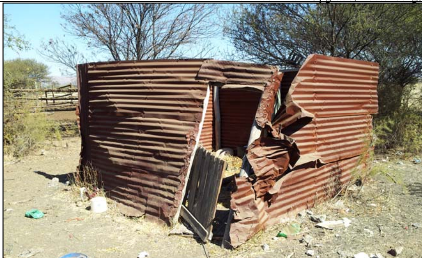
Figure 11: The remains of a dilapidated shelter
