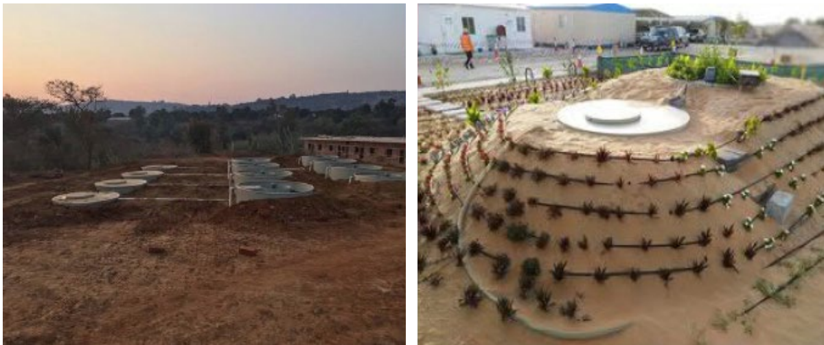
Figure 7: Examples of installed TreeWells
