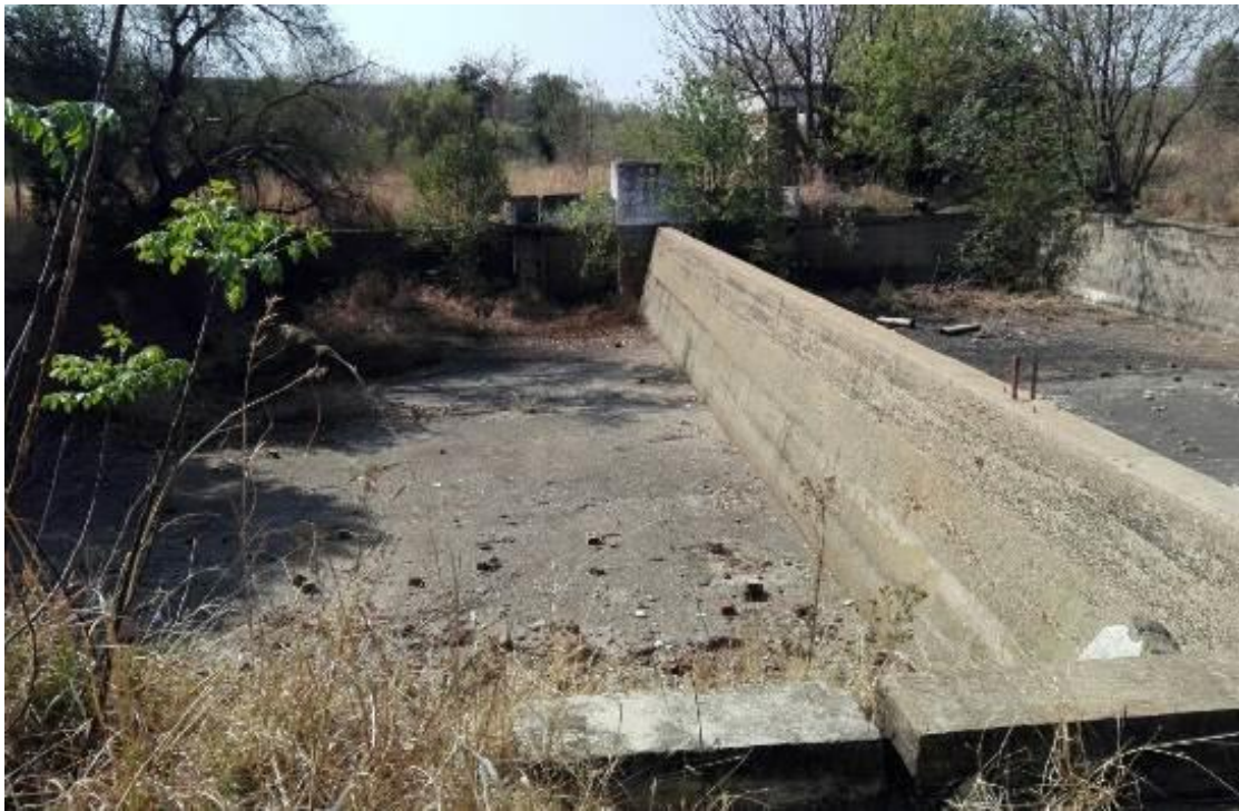
Figure 9: Water reservoirs situated close to power station building
