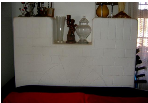
Figure 31. The third fireplace was brick-built, plastered and pointed to imitate a typical Art-Deco fireplace. (Photograph S.M. Miller 2016.)
