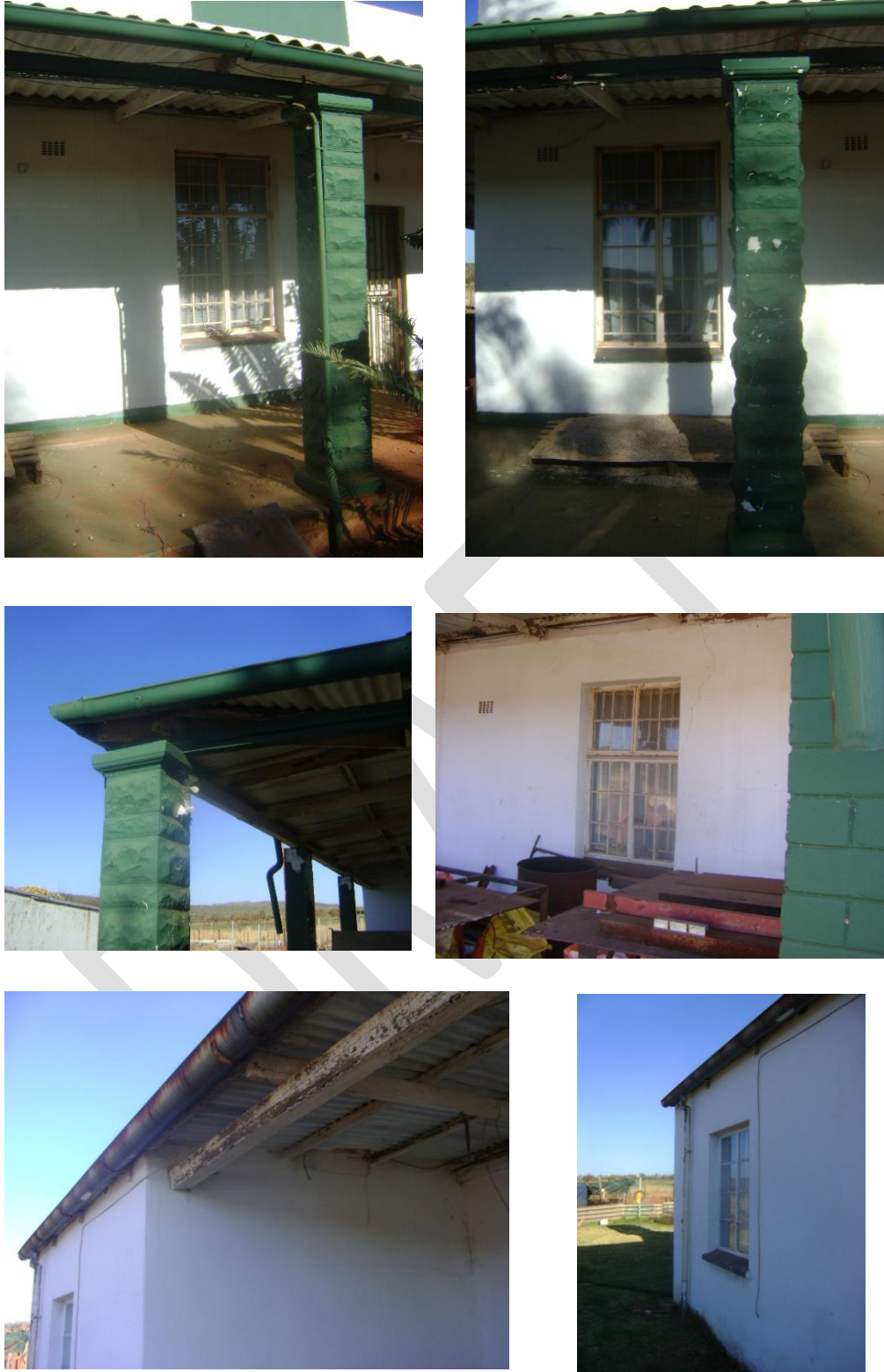
Figure 26. General views of the exterior, elevations and details of the building under investigation. (Photographs S.M. Miller 2016.)
