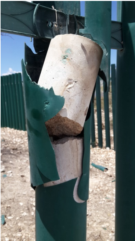
Fig 5: poor execution of concrete mixture – no reinforcement
