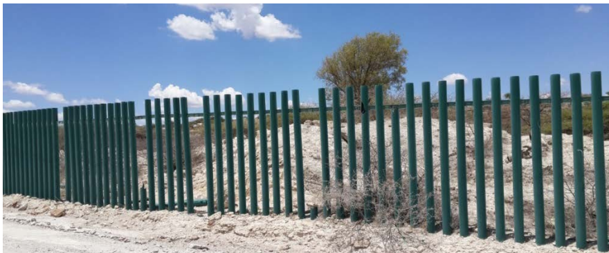
Fig 02 : damages and poles missing on long sections of fencing
