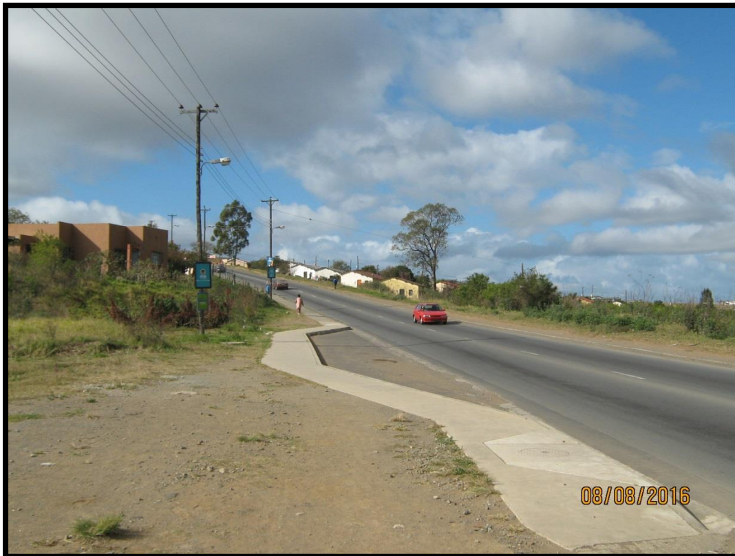
Figure 7: View to show embankment (sandstone) and road, view towards the west. Position of culvert 4.
