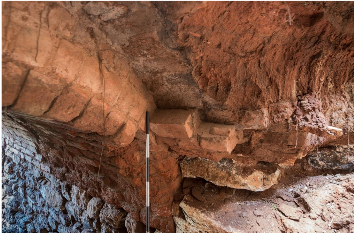
Figure 40. Detail of the joint between the brick vaulting and the kiln base. Note the erosion of the low quality bricks and the frog imprint.
