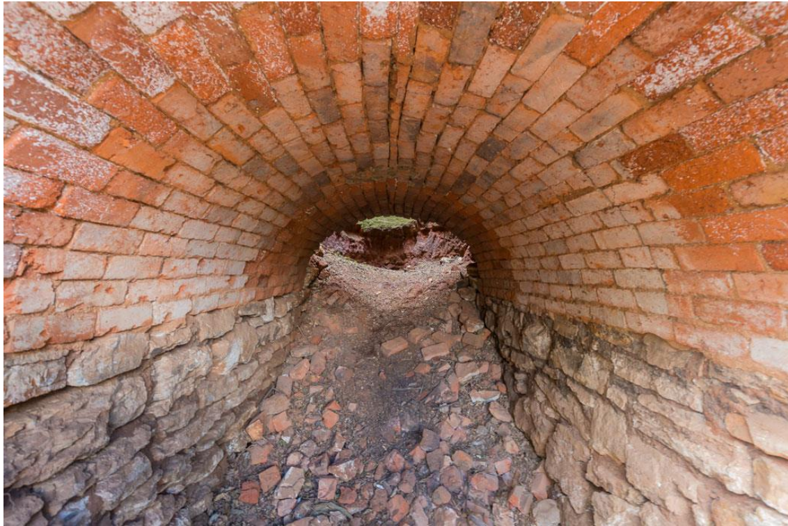
Figure 38. Interior view of the draw hole. Note how the bricks in the top of the arch were cut as key stones.
