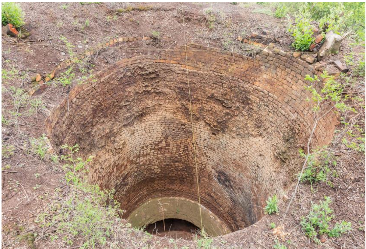
Figure 30. Top view of the southernmost kiln. Note the double brick lining of the kiln and the extensive damage to the brick lining caused by the firing of the kiln. Most of the
