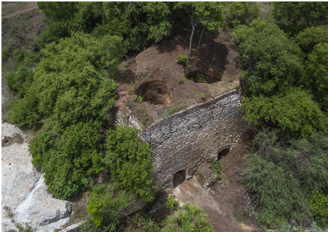
Figure 28. The kilns viewed from the southeast. The eastern wall is the most stable and intact while the southern wall (concealed by trees) had partially collapsed and was repaired at some stage.
