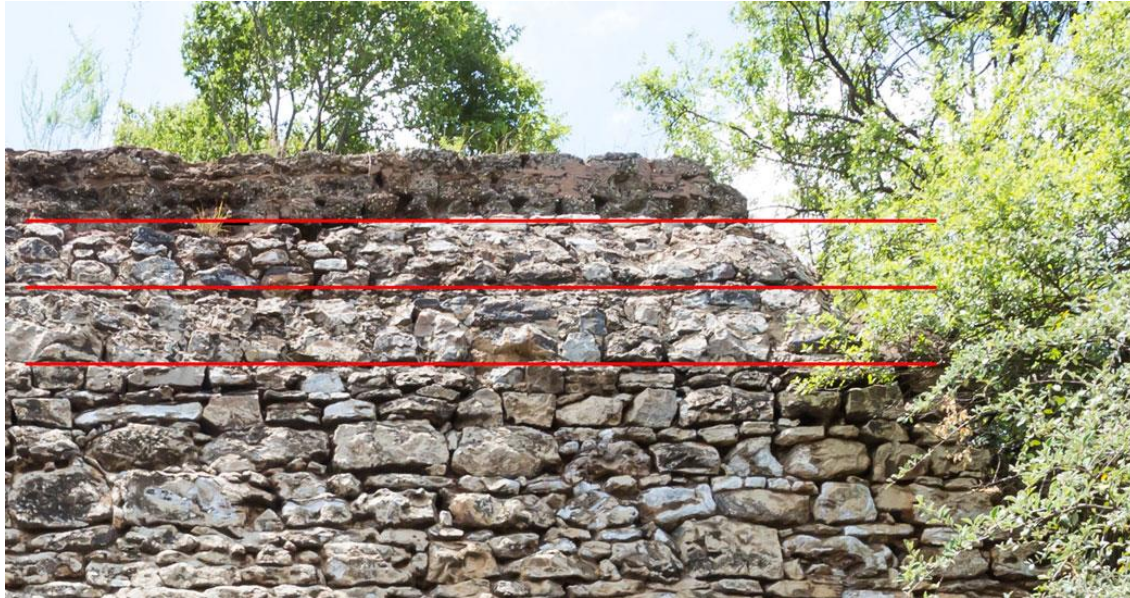
Figure 44. Consecutive raising of the kiln height. Note the original stonework quality versus the two later additions and the lime bricks at the top.
