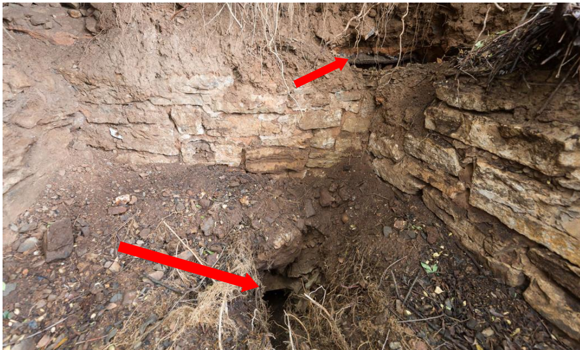
Figure 46. Note the remains of steel railway sleepers in the draw holes.
