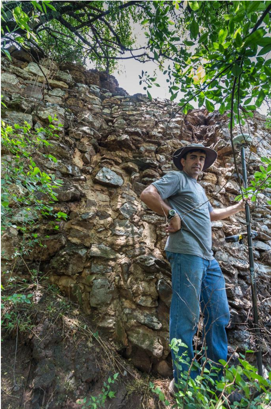
Figure 51. Due to thermal expansion, distortion and the installation of the coal chute the southern wall of the kiln buckled and broke in several places. Note the large section behind the surveyor that was subsequently repaired.
