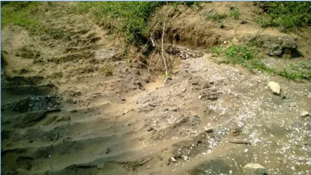
FIG. 7: THE DAMAGE AT MPE 148
