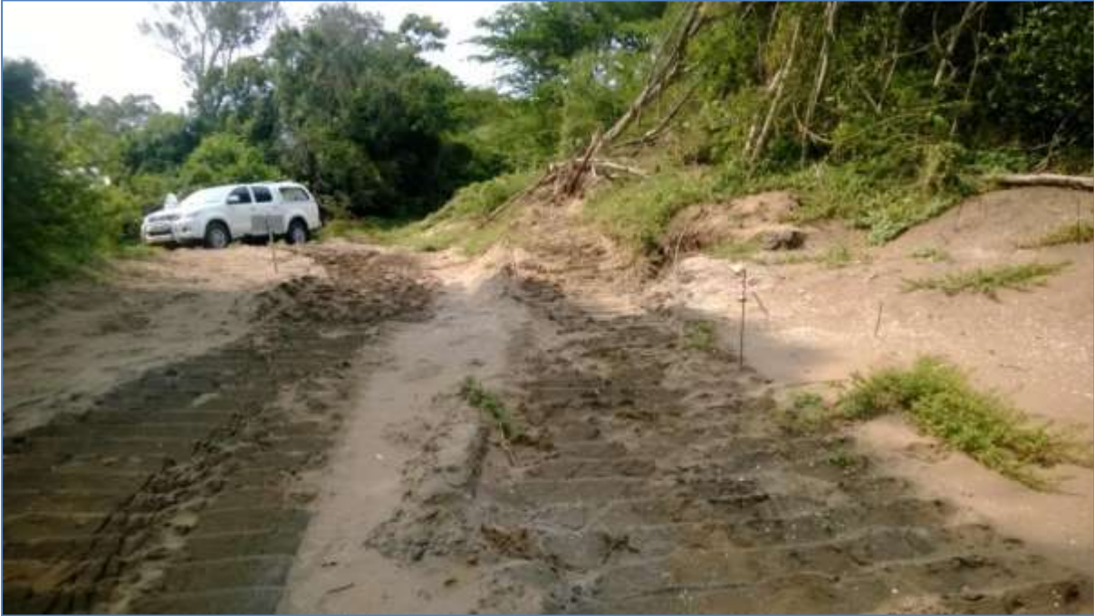
FIG 6: THE DAMAGE AT MPE 148
