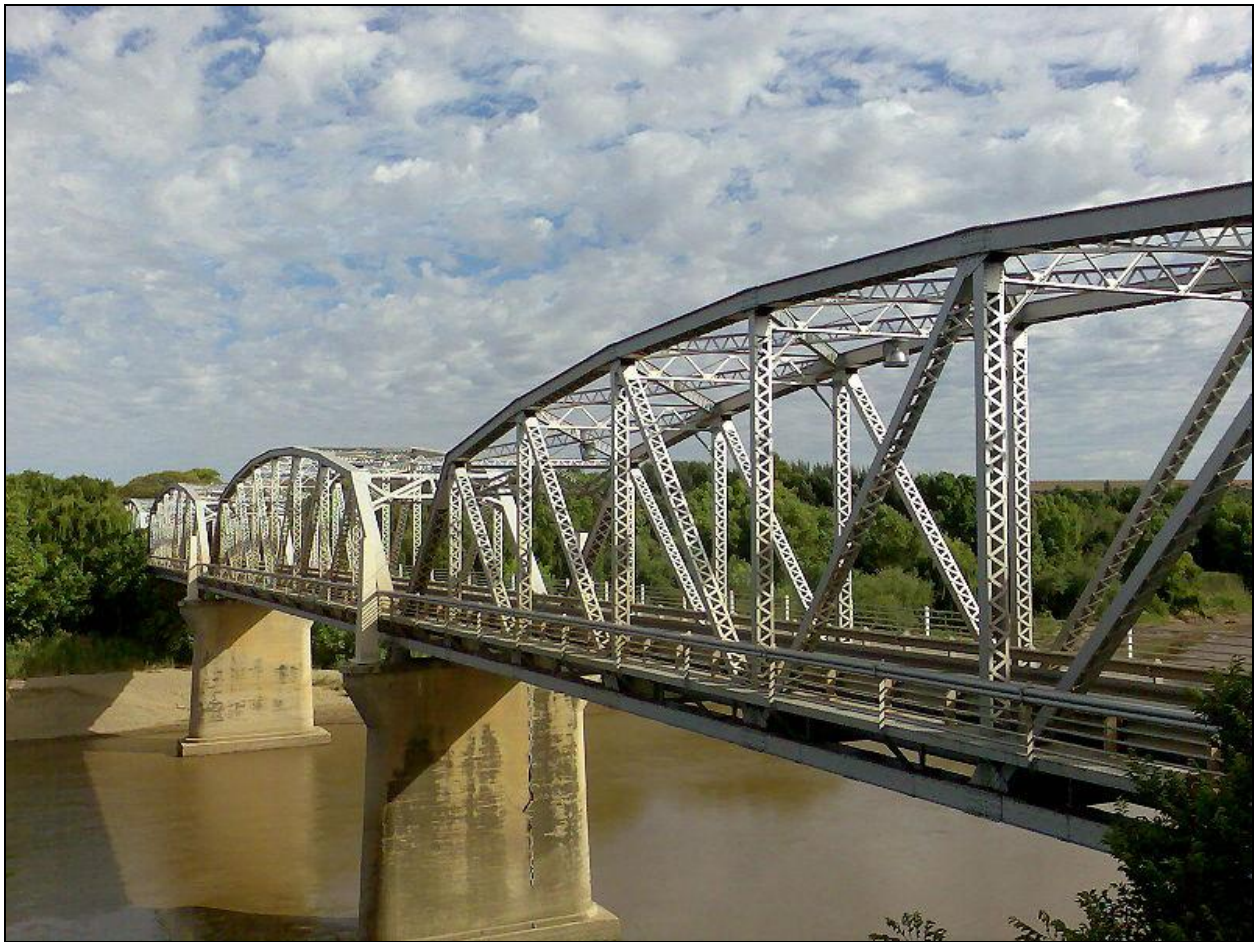
FIGURE 41: Opened in 1937, the Hertzog Bridge across the Orange River at Aliwal North is a landmark protected in terms of Section 34 (older than 60 years) of the NHRA
