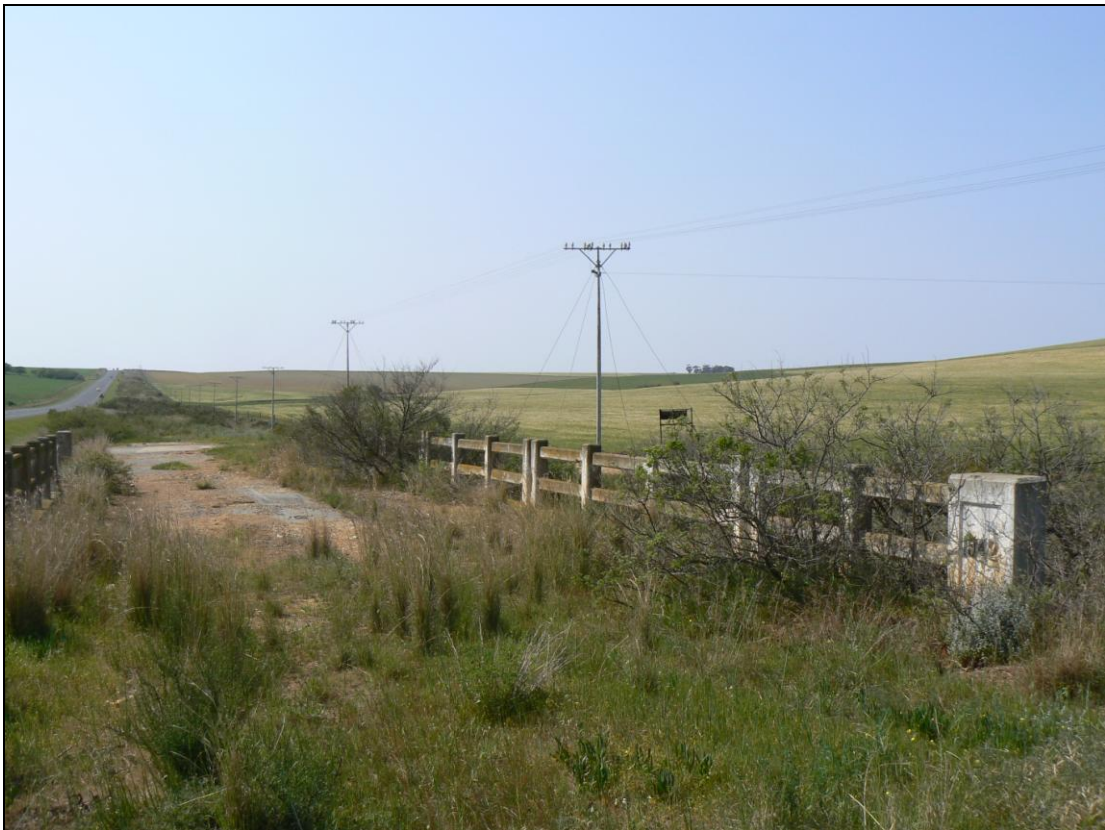
FIGURE 30: Old N 2 alignment between Riviersonderend and Heidelberg with bridges constructed in the mid-1940s
