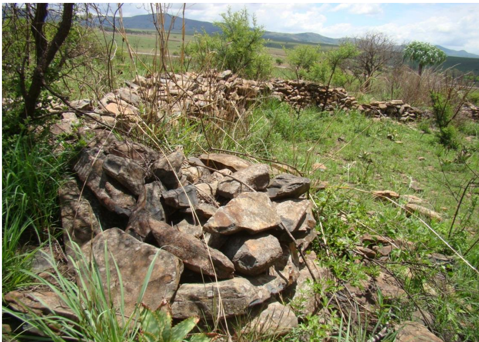
Photo 64: The condition of some of the walls in RDR 1 I.
