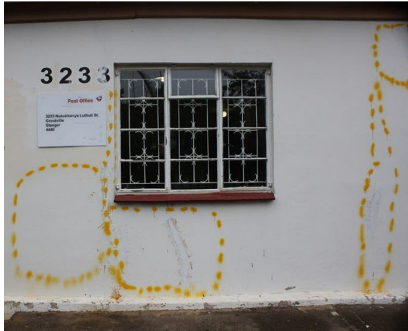
Fig. 8: Marked hollow plaster sections
