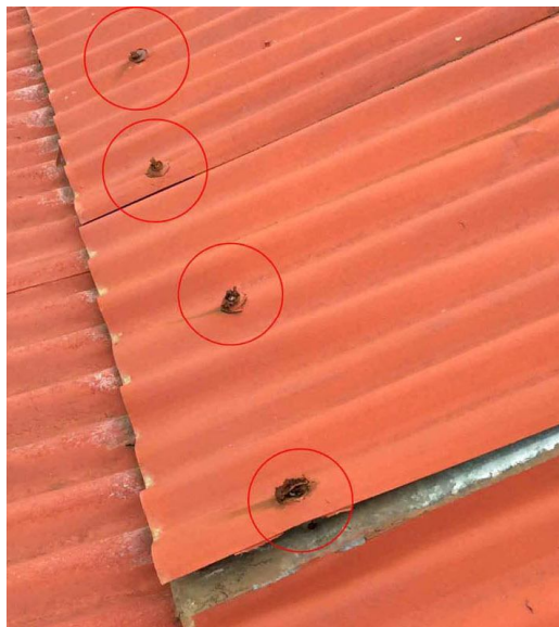
Fig. 1: Loose fixing screws
