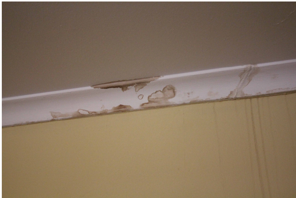
Fig.10: Internal leak probably from air-conditioning unit over.
