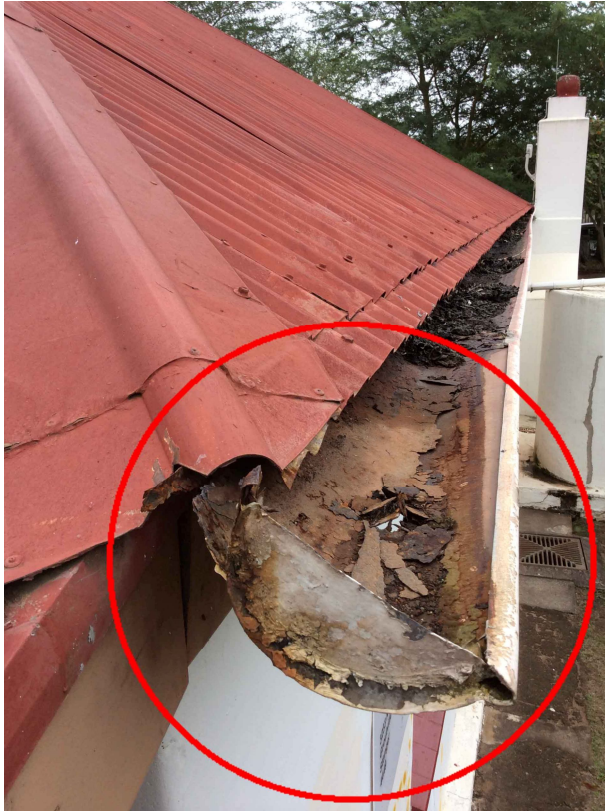
Fig. 6A: Totally corroded gutters!
