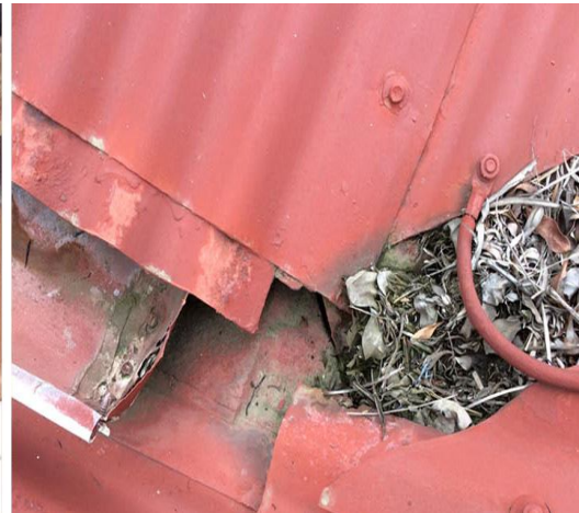
Fig. 4: Gap in flashing evident
