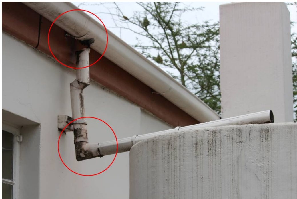
Fig. 5: No connection between gutter and rwdp
