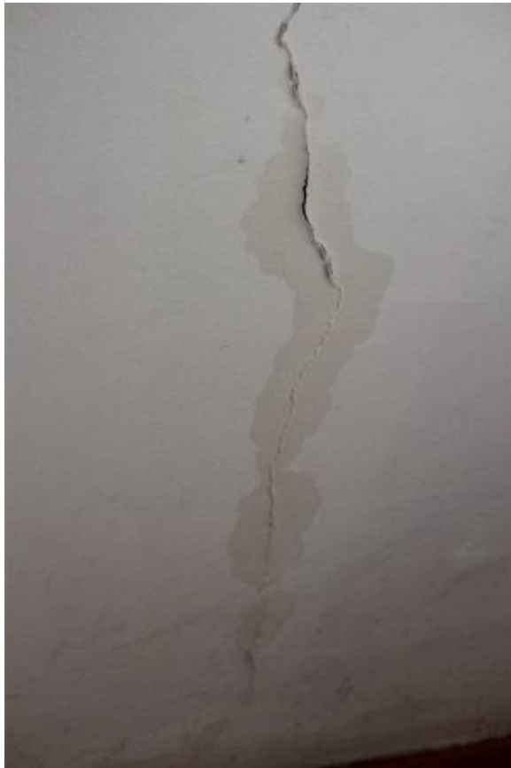
Fig. 13: Minor cracks in concrete plinth
