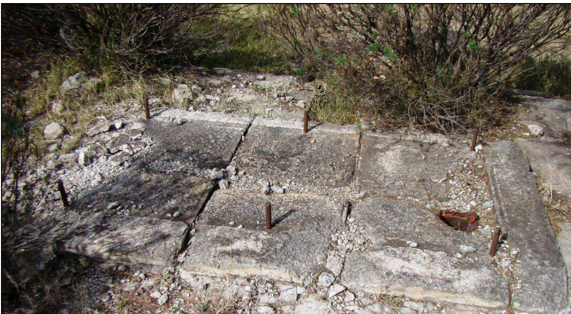
Fig.15 Point R. Remains around bore hole.
