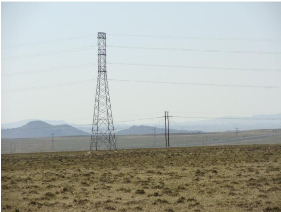
Figure 9: ESKOM power lines in the surveyed area.
