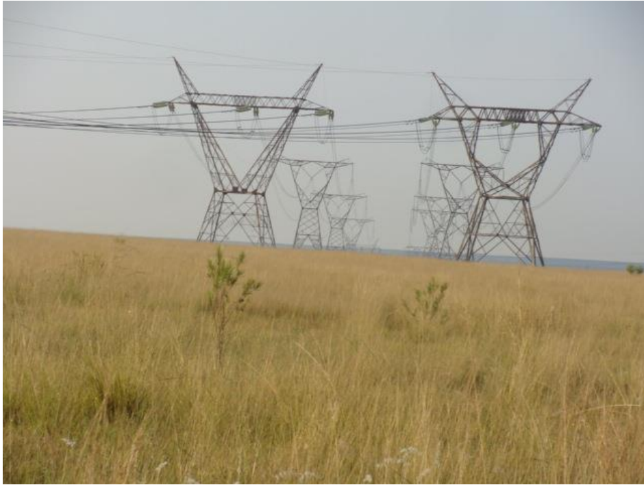
FIGURE 16: VIEW OF VEGATAION AT POINT WHERE THE PROPOSED POWER LINES ROUTE ENDS.
