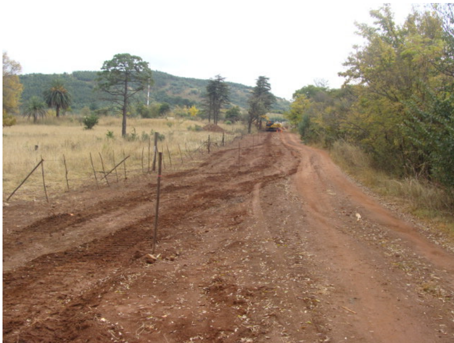
FIGURE 16: GRAVEL ROAD TOWARD THE EAST OF THE TOWN IN THE DIRECTION OF THE WTW, WHERE THE PIPELINE WILL BE INSTALLED.
