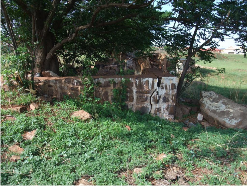
FIGURE 11: ONLY REMAINING STONE WALL THAT MAY HAVE BEEN THE FOUNDATION OF A FARM HOUSE
