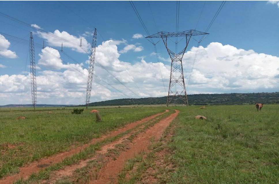
Figure 9: View of high voltage powerlines in the surveyed area.
