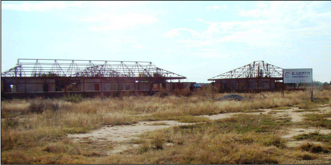
Fig.16 Ransacked structures at the Bothaville ethanol plant site.
