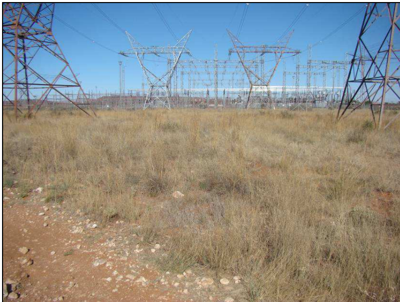
Fig.2 Pylon 1 at Ferrum Sub-station near Kathu.
