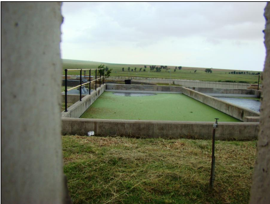
Fig.10 The sewer plant at Glen Lenie, Harrismith.
