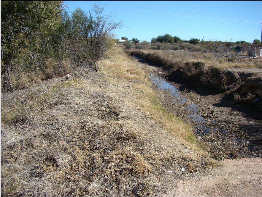
Fig.5. Flood water ditch at Point CK, Melkstroom 563, Upington.
