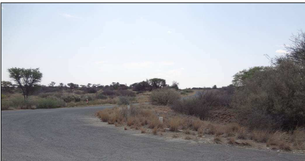
Fig.37 Point V along the Riverton – Boshof – Dealesville water pipeline.
