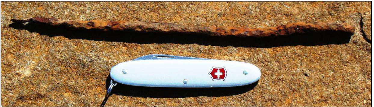
Fig.19 Corroded metal shaft from stone wall site at Point G (Pocket knife = 84mm).
