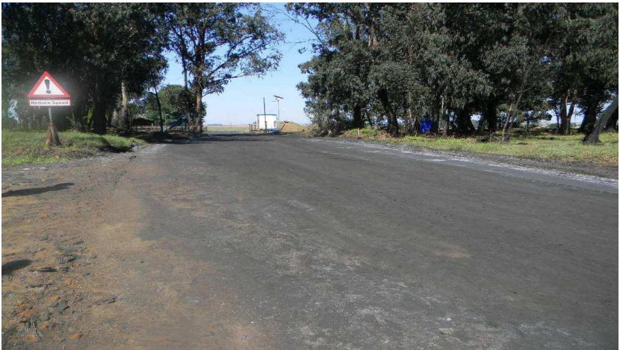
Plate 2: Photo 2: View of the existing road earmarked for upgrading (Photograph © by Author 2017).
