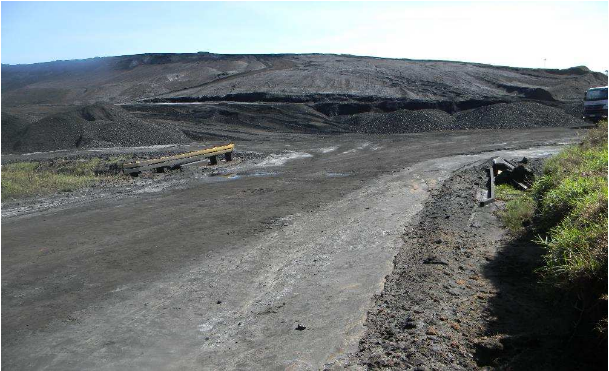
Plate 1: Photo 1: View of Matla Coal stockpile site where the proposed road will start (Photograph © by Author 2017).
