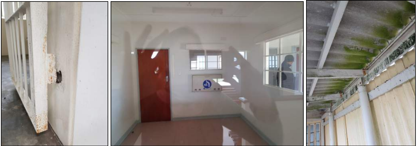
Figure 4.3, 4.4 and 4.5: Visitors Centre - Although recently restored, maintenance is required as well as the removal of insensitive modern additions such as changing table
