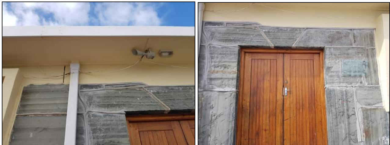
Figure 3.8 and 3.9: Murray Harbour Office - Inappropriate electrical infrastructure and pointing requires maintenance
