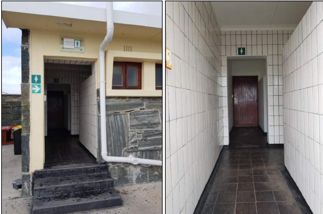
Figure 3.10 and 3.11: Murray Harbour Office - Toilets: Previously separate entrances for white people and black people, walls broken down to increase toilet size
