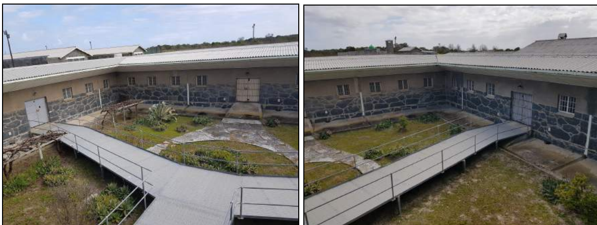
Figure 5.17 and 5.18: Prison Precinct - Inappropriate Universal Access ramps in hospital courtyard
