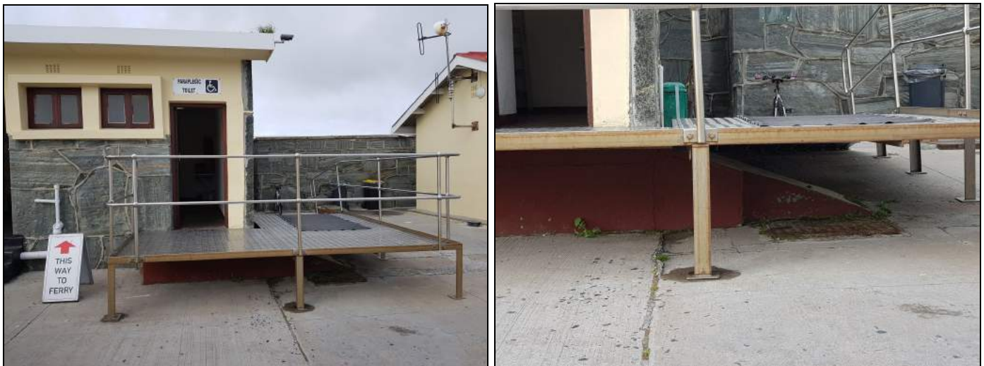
Figure 3.12 and 3.13: Murray Harbour Office - Intrusive and inappropriate universal access ramps for toilet access placed over existing ramp
