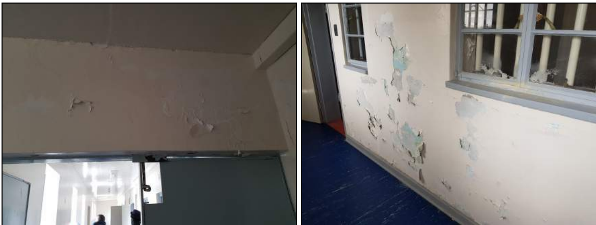
Figure 5.15 and 5.16: Prison Precinct - Hospital wing requires maintenance
