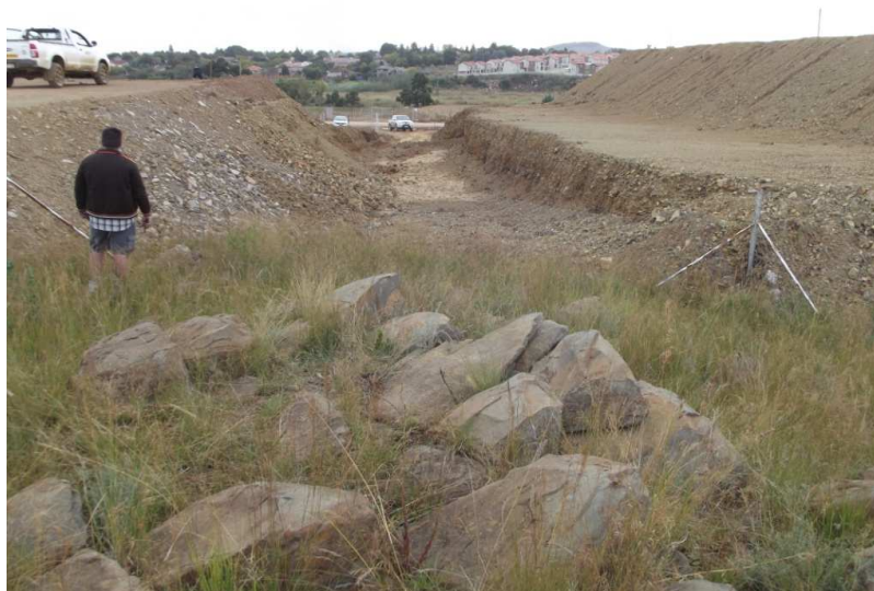
Fig. 3: Current view of the area after construction has commenced. Access was extremely difficult.
