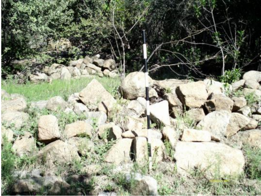
Figure 131: Another collapsed stone wall.
