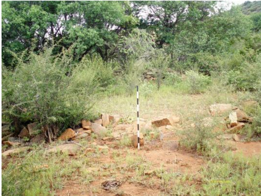
Figure 25: Collapsed stone wall.
