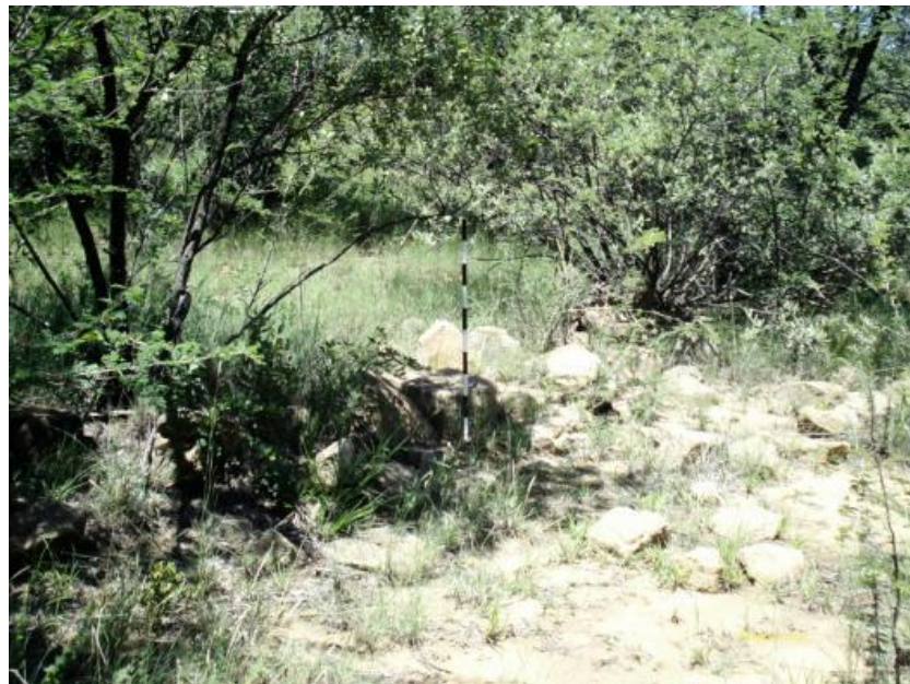
Figure 110: Another collapsed stone wall.
