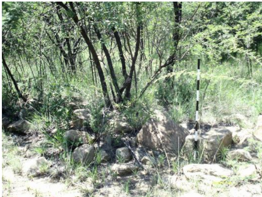
Figure 112: Stone wall that is overgrown with vegetation.
