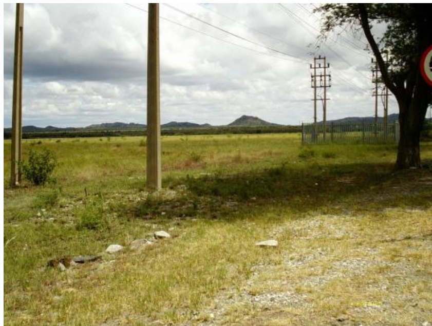
Figure 3: Power lines running along the site.
