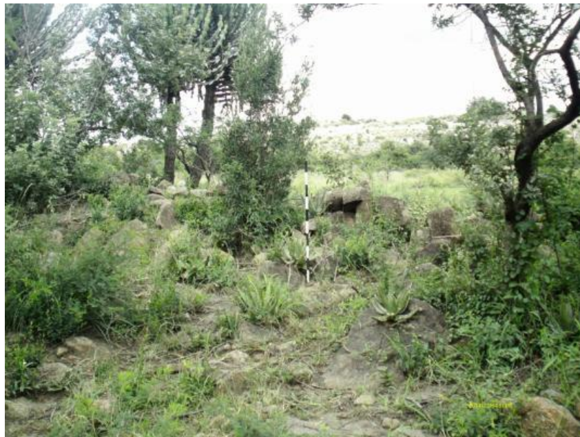
Figure 93: Collapsed and overgrown stone wall.
