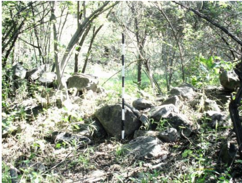
Figure 130: Collapsed stone wall.
