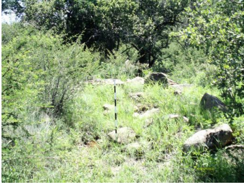
Figure 1: A collapsed and low stone wall.
