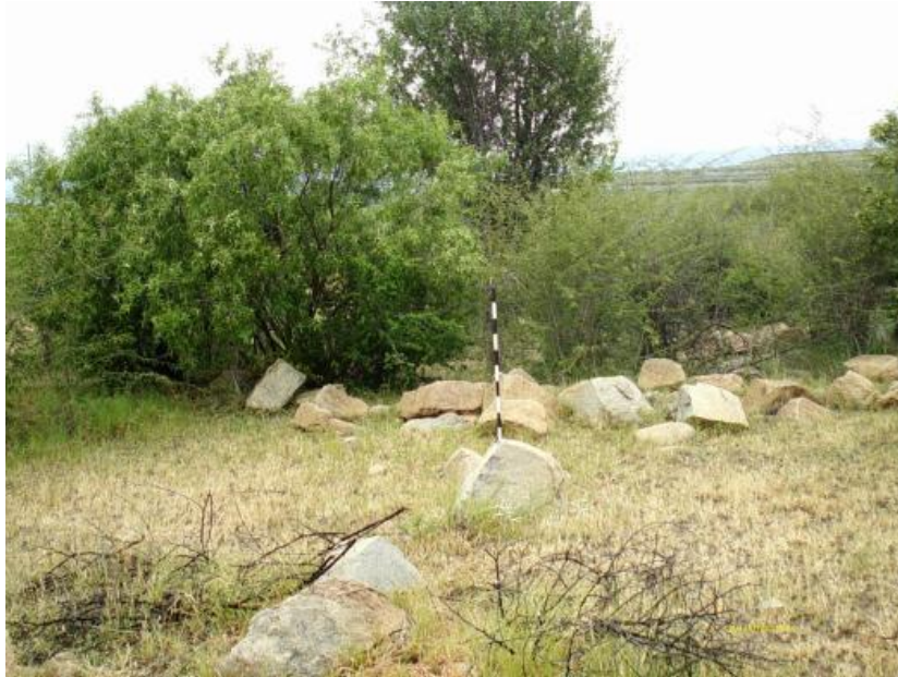
Figure 54: Collapsed stone wall.
