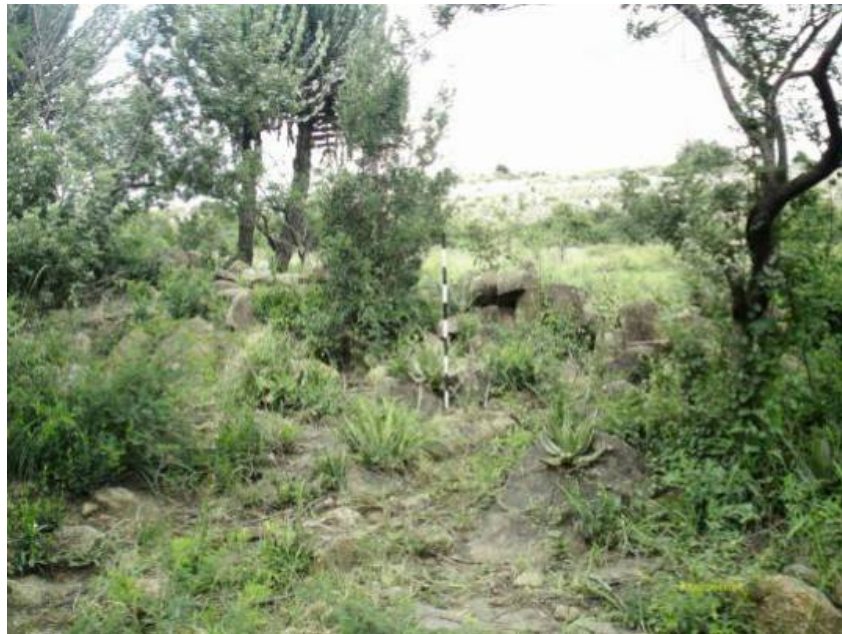
Figure 93: Collapsed and overgrown stone wall.
