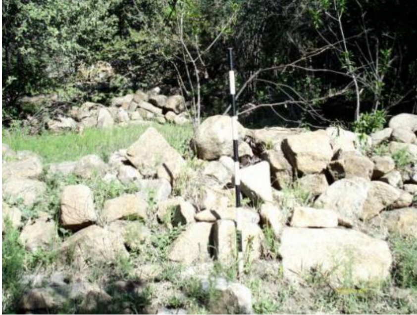
Figure 131: Another collapsed stone wall.
