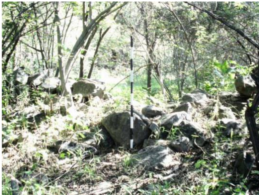
Figure 130: Collapsed stone wall.
