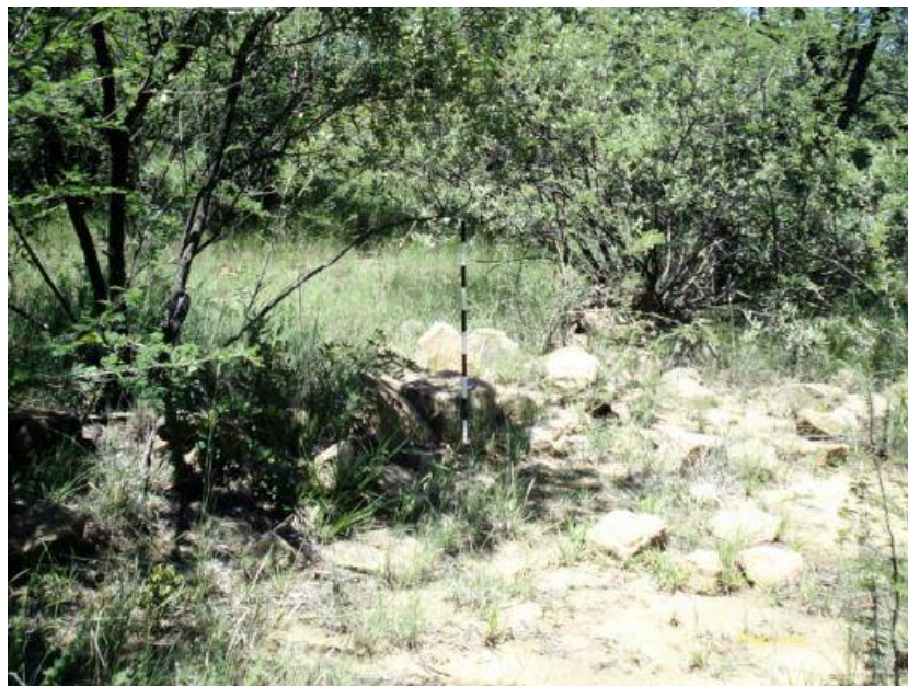
Figure 110: Another collapsed stone wall.
