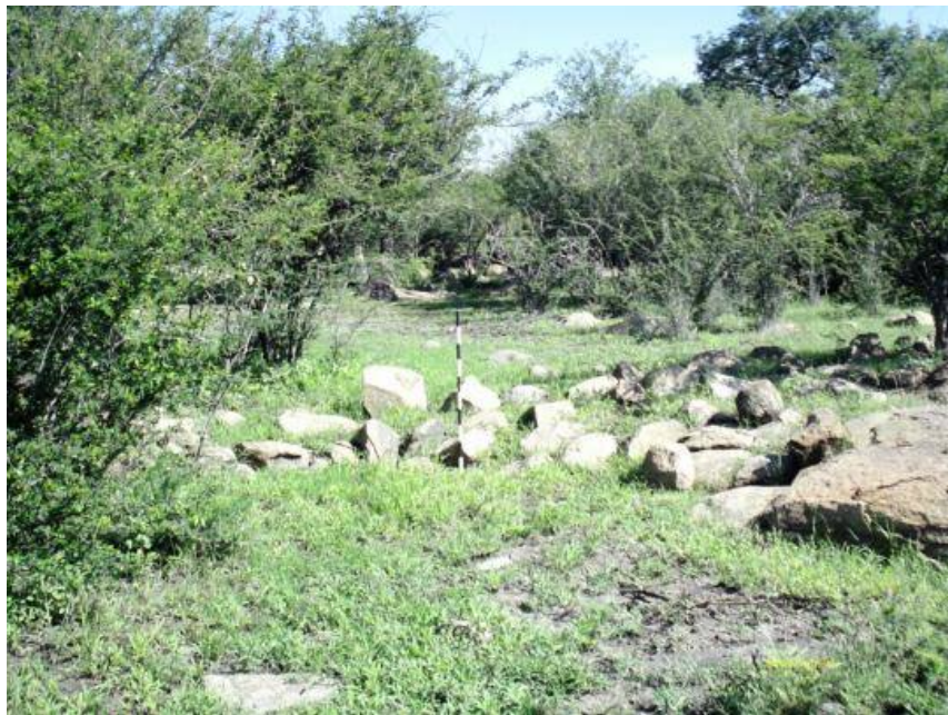
Figure 124: Collapsed Stone wall on site.
