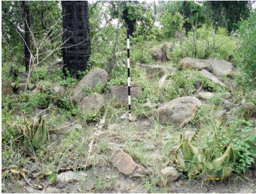
Figure 92: Collapsed stone wall.
