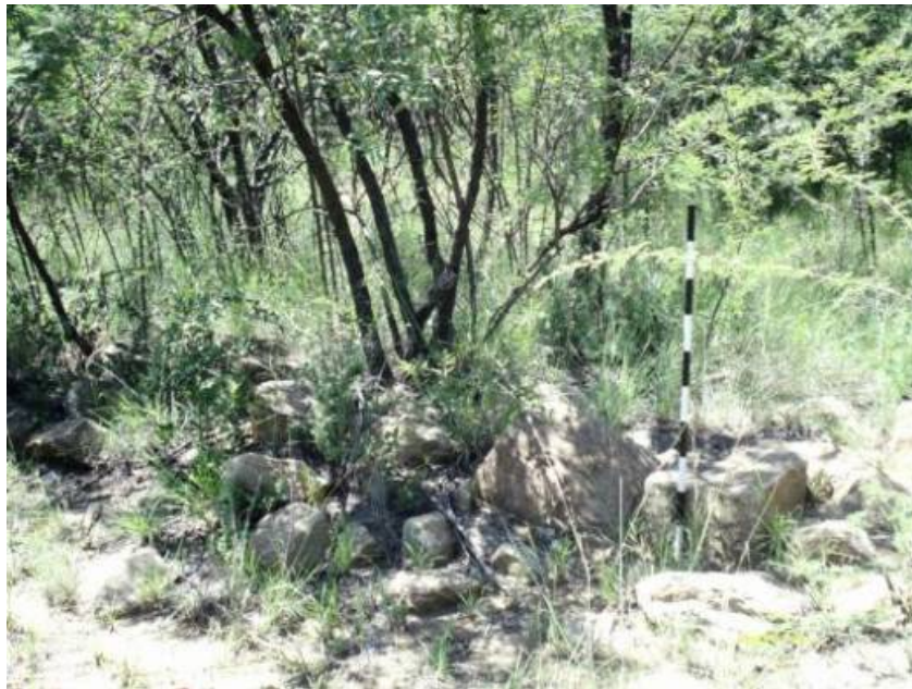
Figure 112: Stone wall that is overgrown with vegetation.
