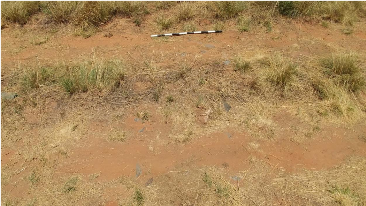
Figure 24: Grave in centre of dirt road.
