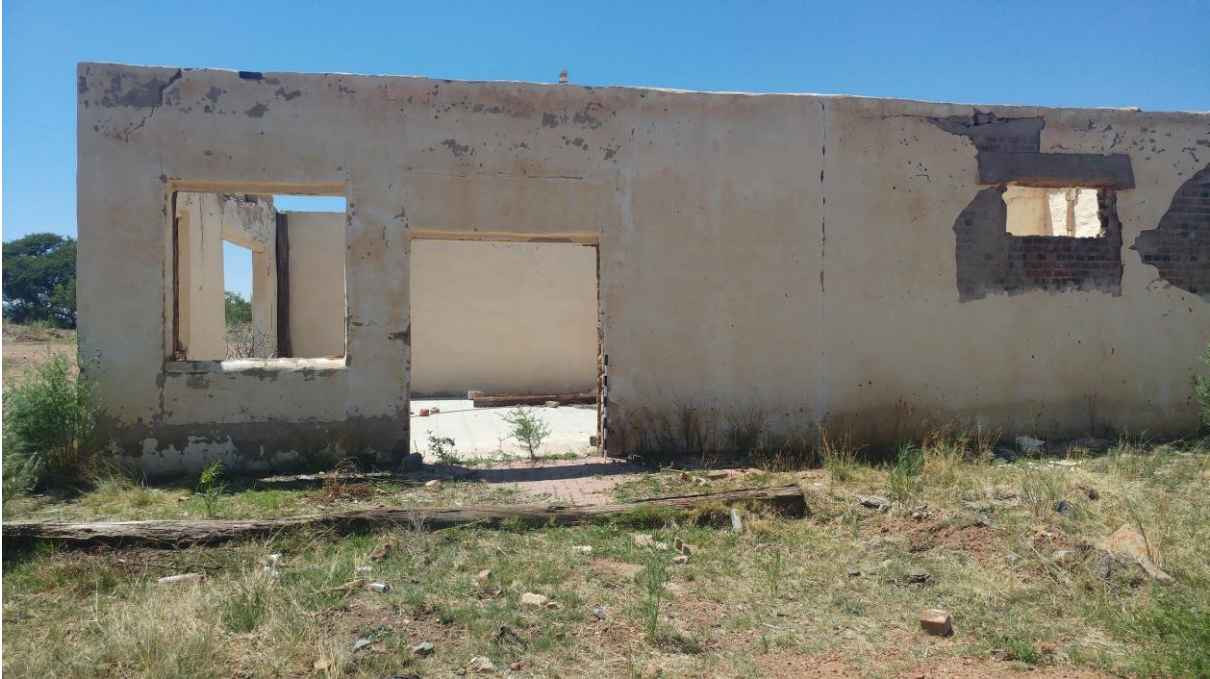
Figure 9: Example of one of the buildings on site which is younger than 60 years of age.
