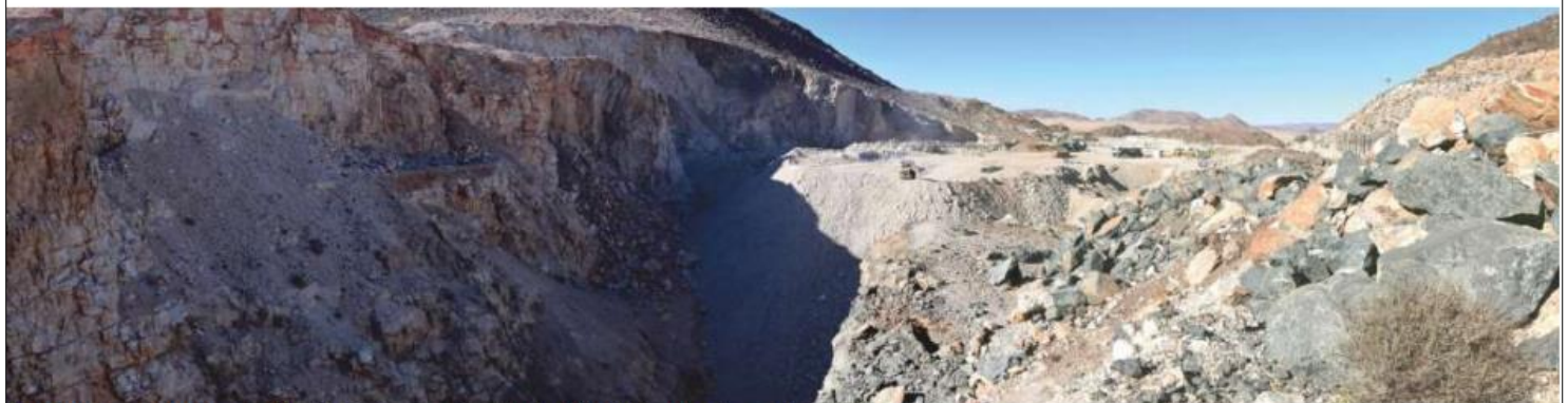
Photo 2: Looking west from the top of the Main Section excavation at the backfill which has taken place to date.
