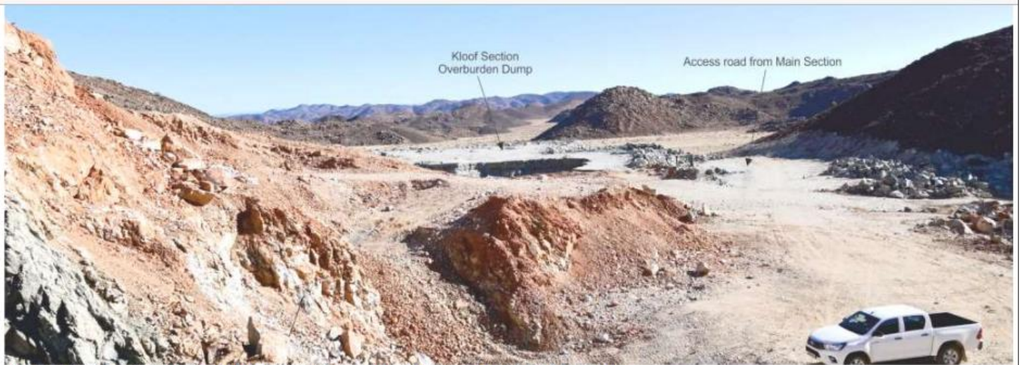
Photo 5: Looking north from the adit of the Kloof Section excavation at the main section access road and the existing waste dump.
