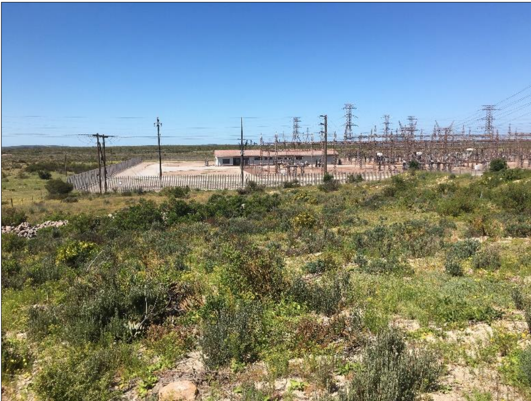
Figure 5. The Blouwater substation (Kaplan 2020).
