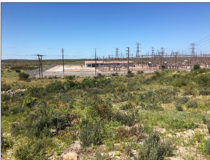
Figure 4. The Blouwater substation.
