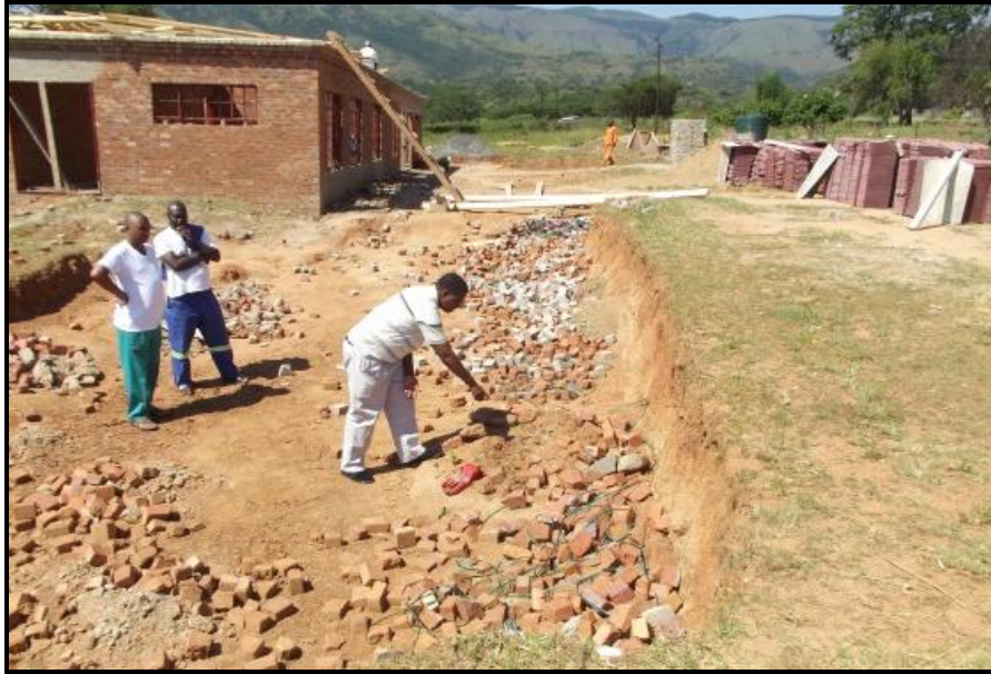
Figure 1. Barberton Museum employee, Mr Julius Matsebula, points to where the human remains were found during excavation activities.
