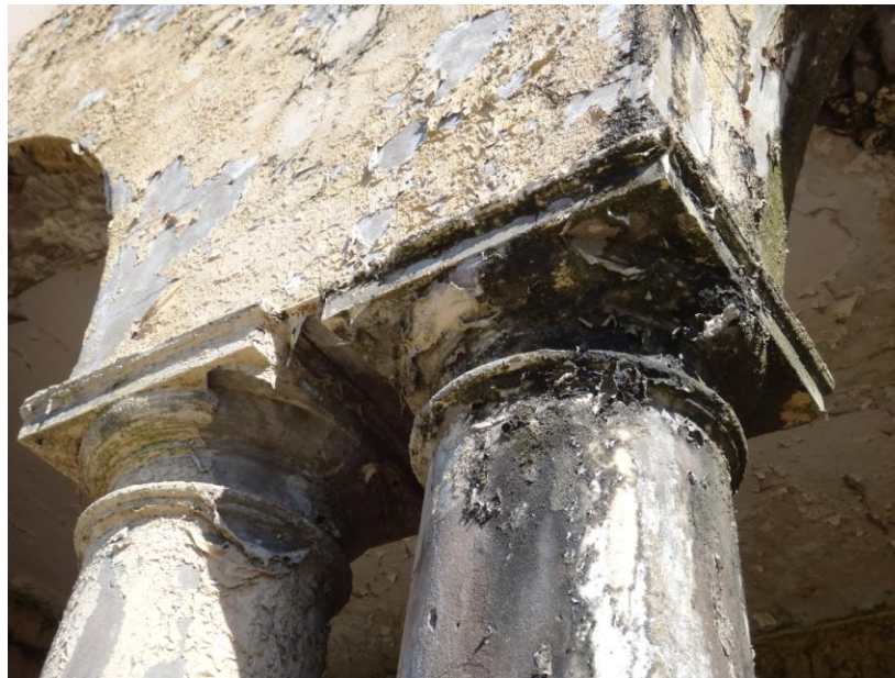
Damaged and chipped Tuscan Doric columns to be repaired.
