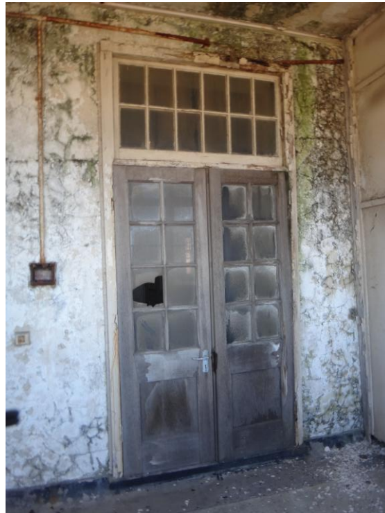
French teak glazed door to veranda, to be repaired where possible.
