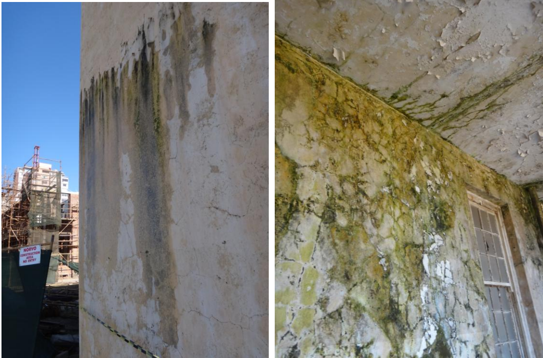
Damage to walls caused by water ingress.
