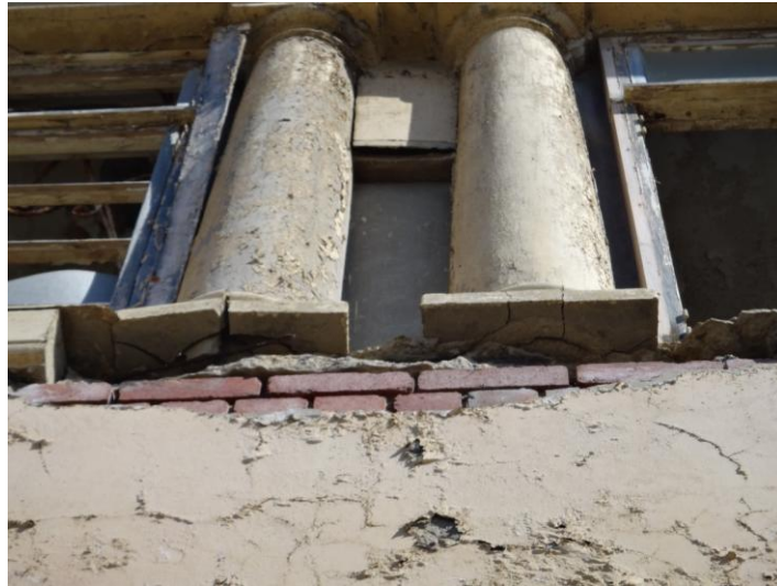
String courses to be replaced where rotten or where they have fallen off.
