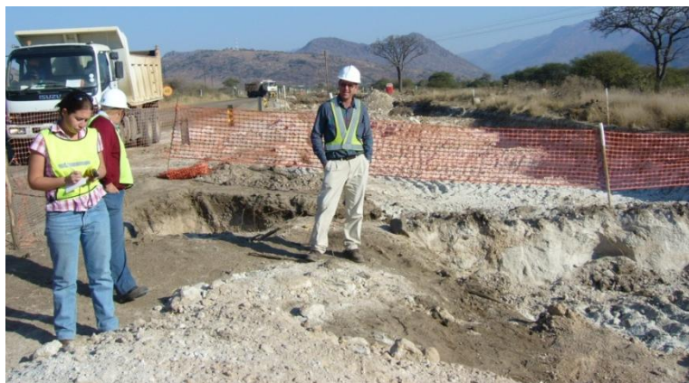
Figure 2. The excavation of the new Richmond road by the construction team, right next to the existing road. The skeletal remains were dislodged by the mechanical equipment.
