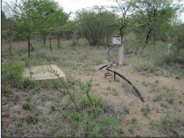
Figure 5: View of the borehole and pump on southern side of the study area.
